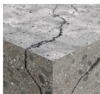
Cracked concrete C20/C25 to C50/C60
